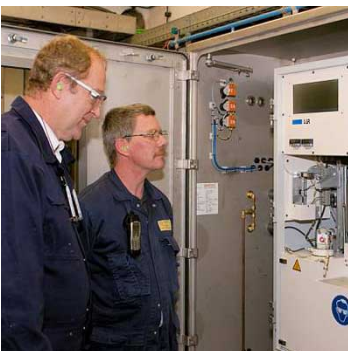
Analyser inspection and application fine tuning
