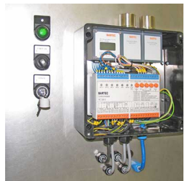
The purge air control unit
