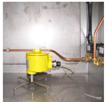
An FCI level switch shuts off the sample pump in case of a leakage
