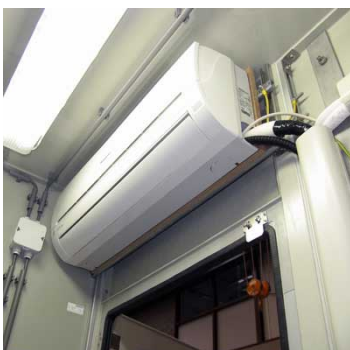
An air conditioner split unit is part of the analyser house package
