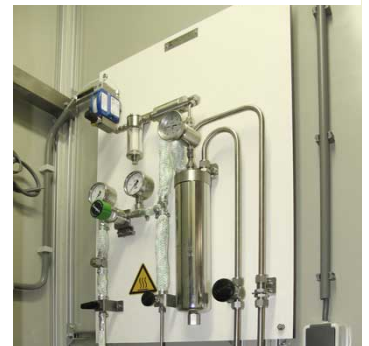
Sample conditioning panel to reduce temperature and pressure
