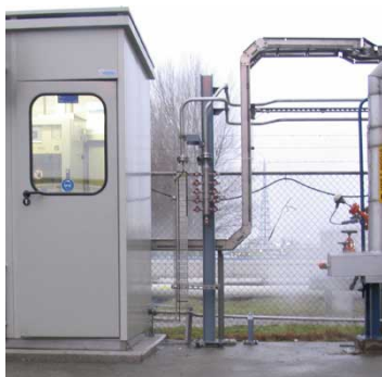
The sample line is only 1/4 " OD and is supported via a duct
