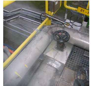
Hot condensate return water is pumped to the boiler
